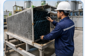
FILL MEDIA CLEANING
